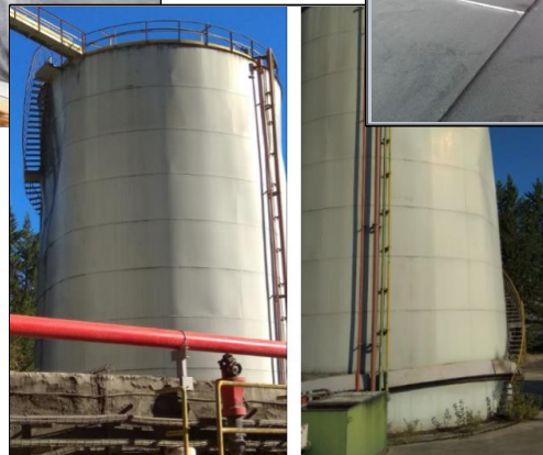
Forensic Engineering | API 650 Storage Tank Failure
